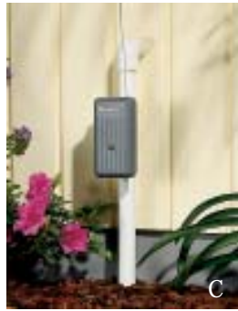
A) Typical indoor installation of SRR receiver unit.
